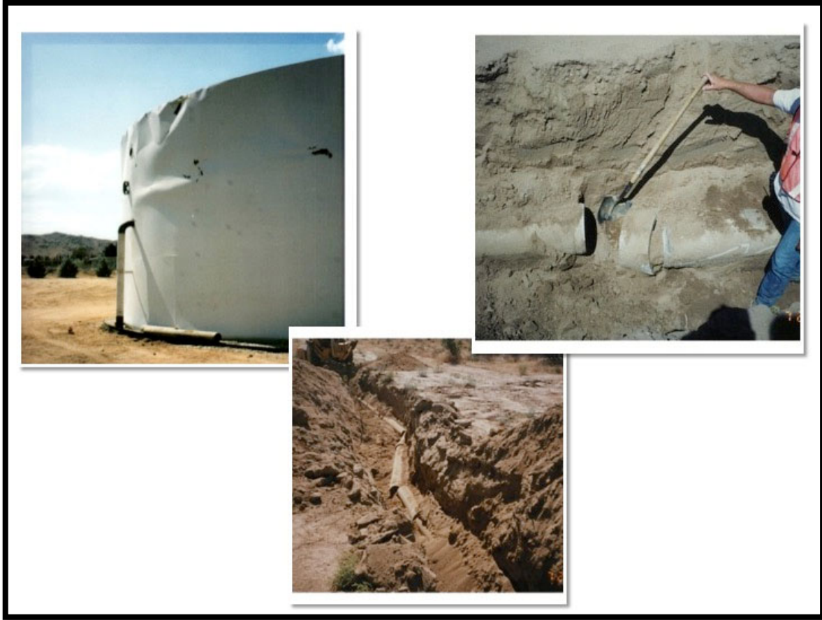
Figure 2 Examples of Earthquake Damage to Water Utility Facilities These examples were from the 1992 Landers Earthquake
